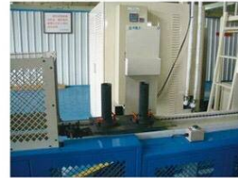
Outer Shell & Inner Tube Loading Station 內外管放入站
